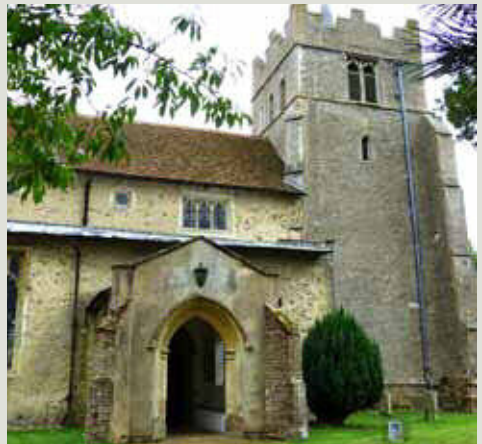
A grant of £4,000 helped All Saints, Ashdon make stonework and plaster repairs.
